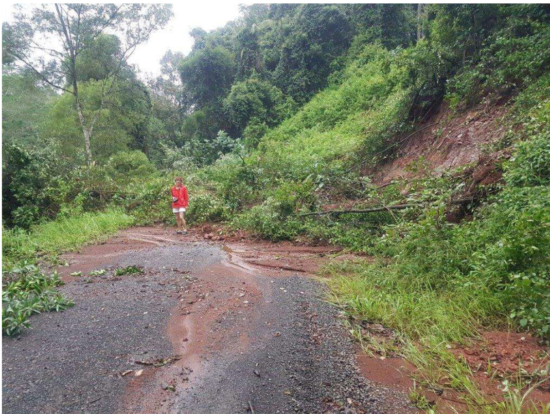
Landslip at Terania Creek Road
